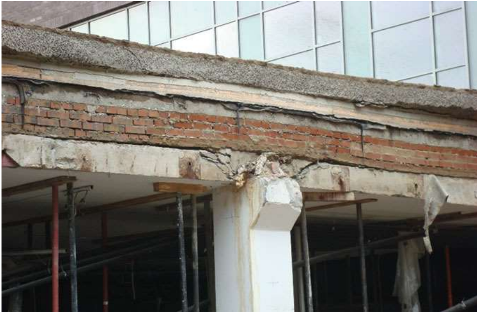
Fig. 4 Flat slab after punching failure
